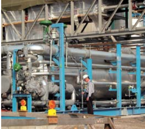
The Detroit Edison Monroe Reactor.
