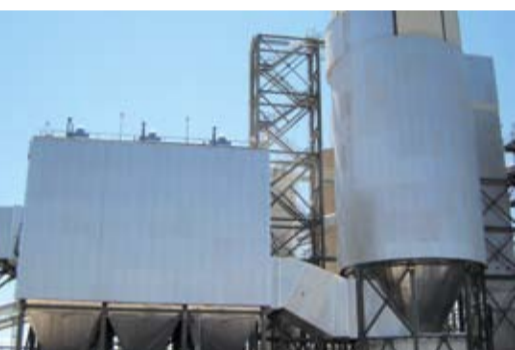
Rocky Mountain Power, baghouse and scrubber.
